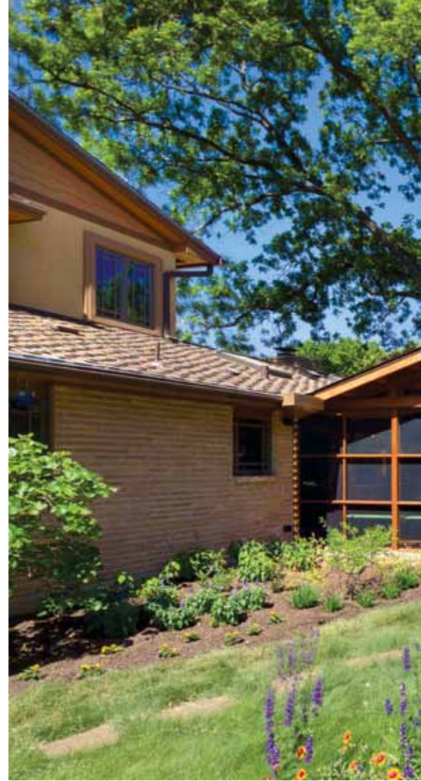
Given the existing house and location of the addition, its roof in effect is a “butterfly” in form. Drainage of this roof required the construction of a “cricket” at the backside of the butterfly. The resultant concentration of water is gathered at the fascia of the existing house with custom-designed rainwater-collection boxes.
